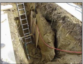
Slough or Belly Failure
